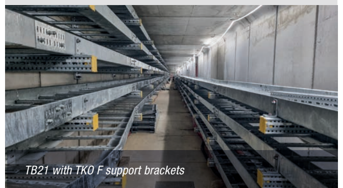
siFramo supports in the Tokamak building
